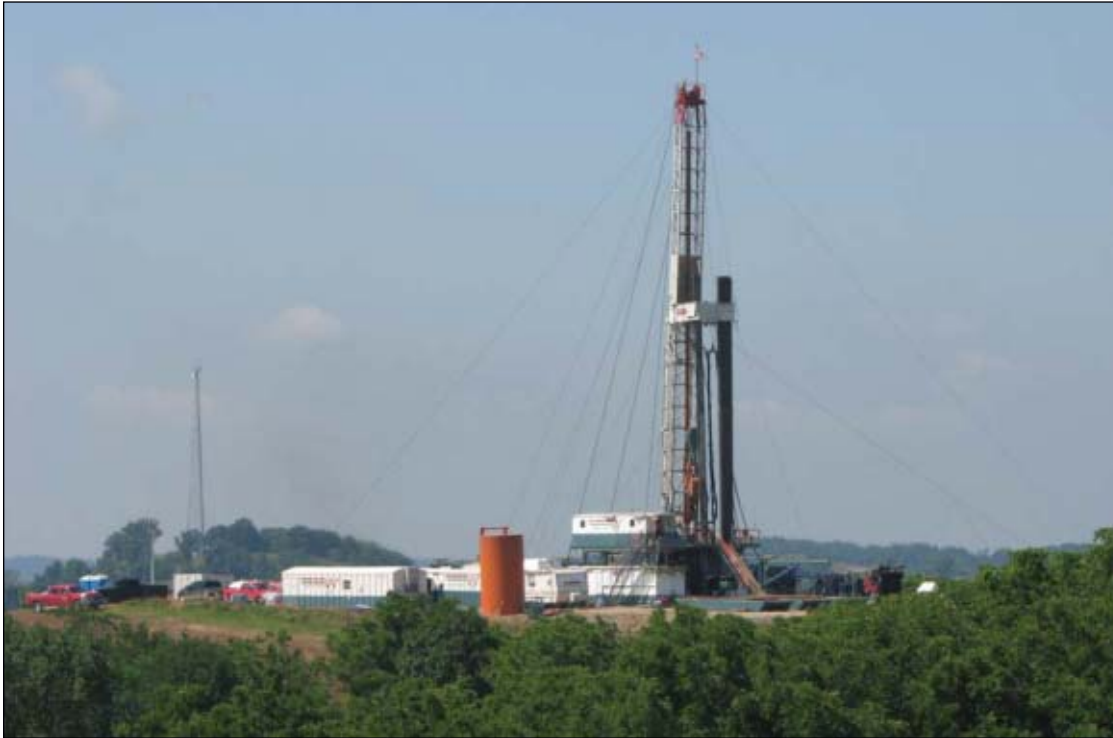
Les Wilson Rig 25 drills the CNX No. 3 well, CNX Gas's first horizontal Marcellus shale well, which began producing at a rate of 6.5 MMcf/d in December (Fig. 2; photo by Harry Giglio from CNX Gas Corp.).
